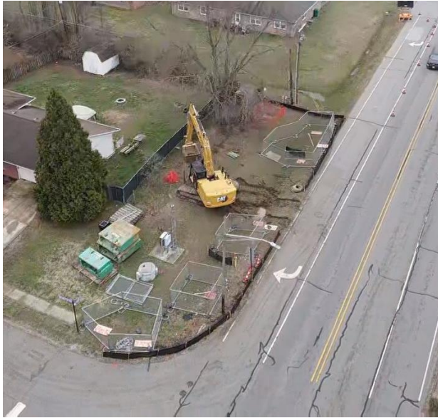
Hyde Park lift station March
